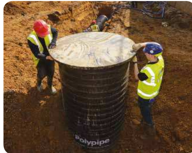
Polypipe delivers a unique earth tube project as part of the redevelopment of Westbrook Primary School
