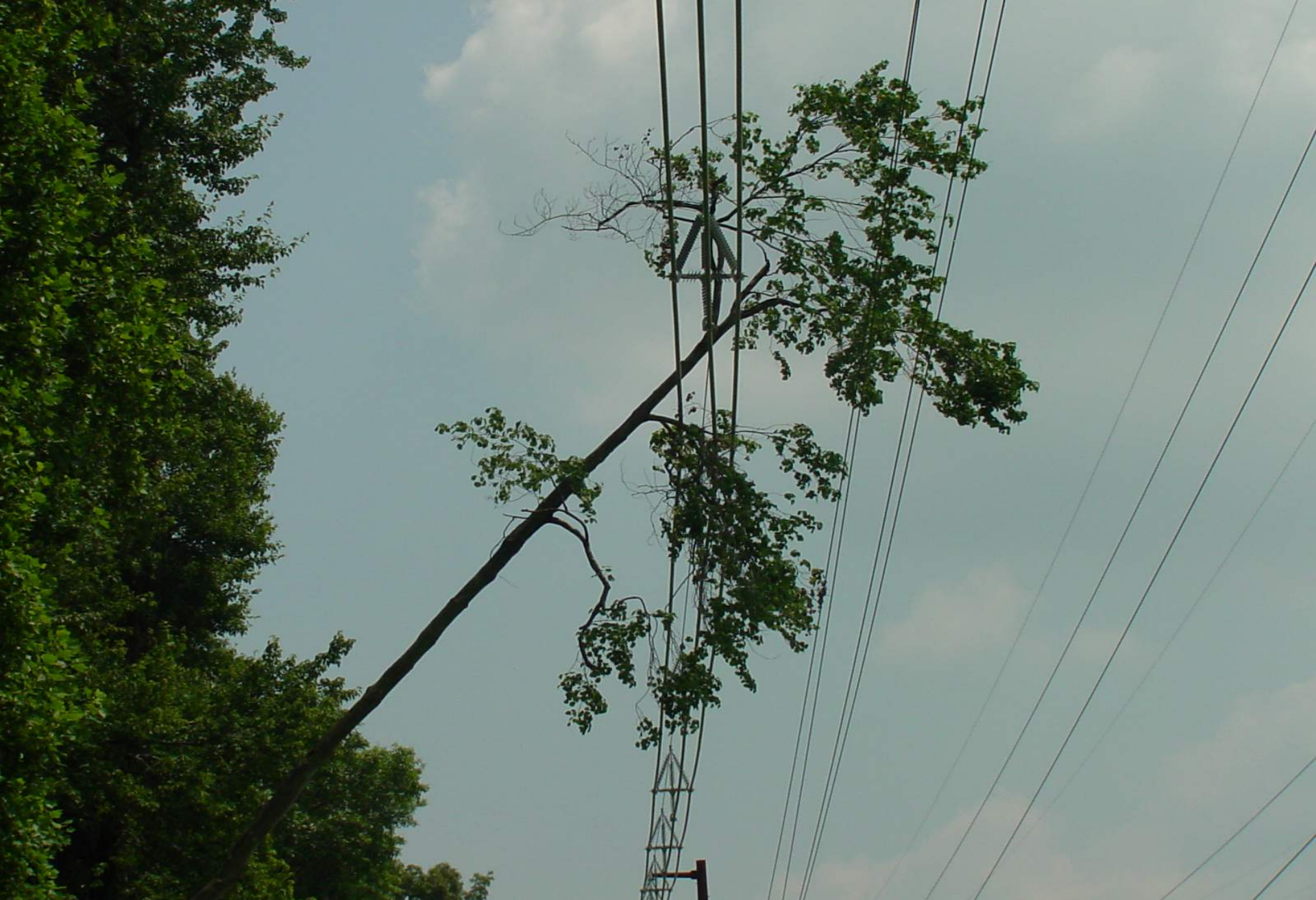
69 kV Spacer Cable PEPCo - Washington, DC
