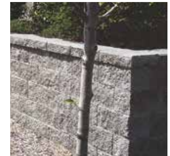
Keystone retaining wall in Flint finish
