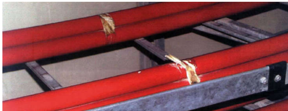
Bundling with fibre-glass reinforced bundling adhesive tapes, functional breakdown of the tapes due to ageing
