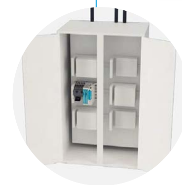
Decentralised power distribution
